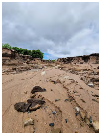
Extensive earthworks are required to make repairs
